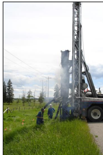
Drilling a groundwater monitoring well south of the Highway 22 bridge crossing the Elbow River.
