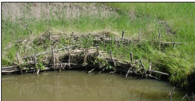
Live reinforced earth wall on the outer bank of a bend at McLean Creek.
